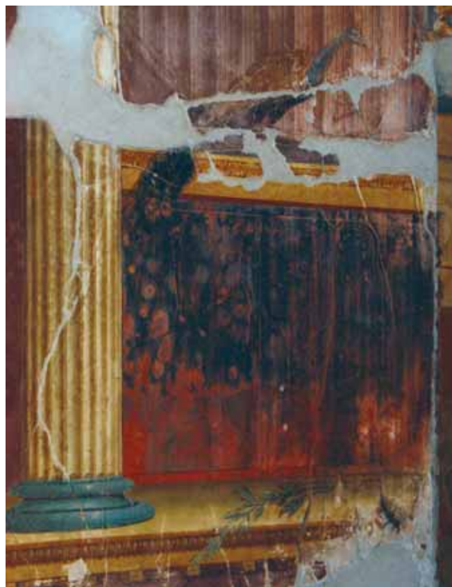
A wall showing the heavy damage due to blackening of cinnabar in the Poppea's villa in Oplonti
