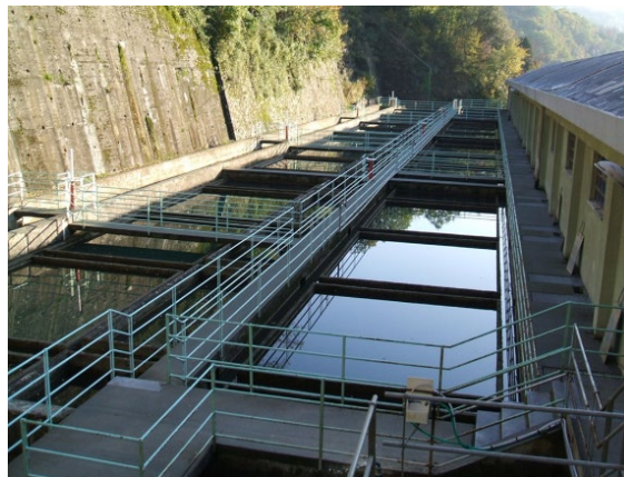
Genoa drinking water treatment © IREN
